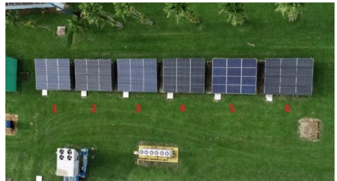
Fig. 6. Aerial photograph of the photovoltaic installation, where each string is identified.
